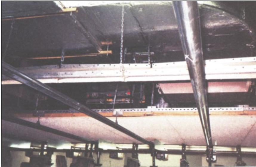
Ductwork for supply air in ceiling.
