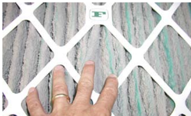
Filter Test: The 30/30 after only four months of operation.
