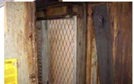
Caramelization on HVAC
